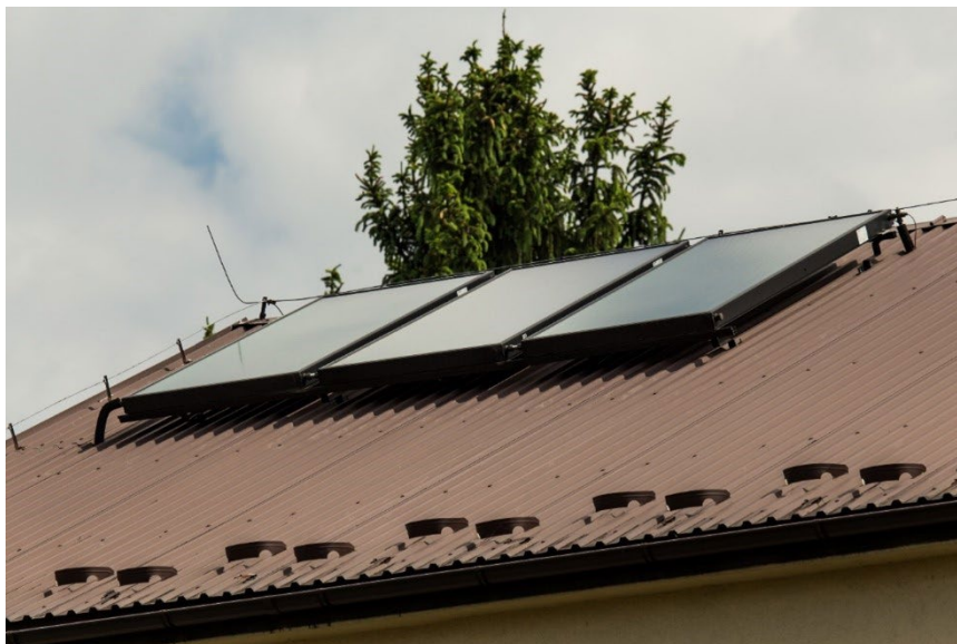
Fig. 1. The flat plate collector installation in detached house Source: own study
