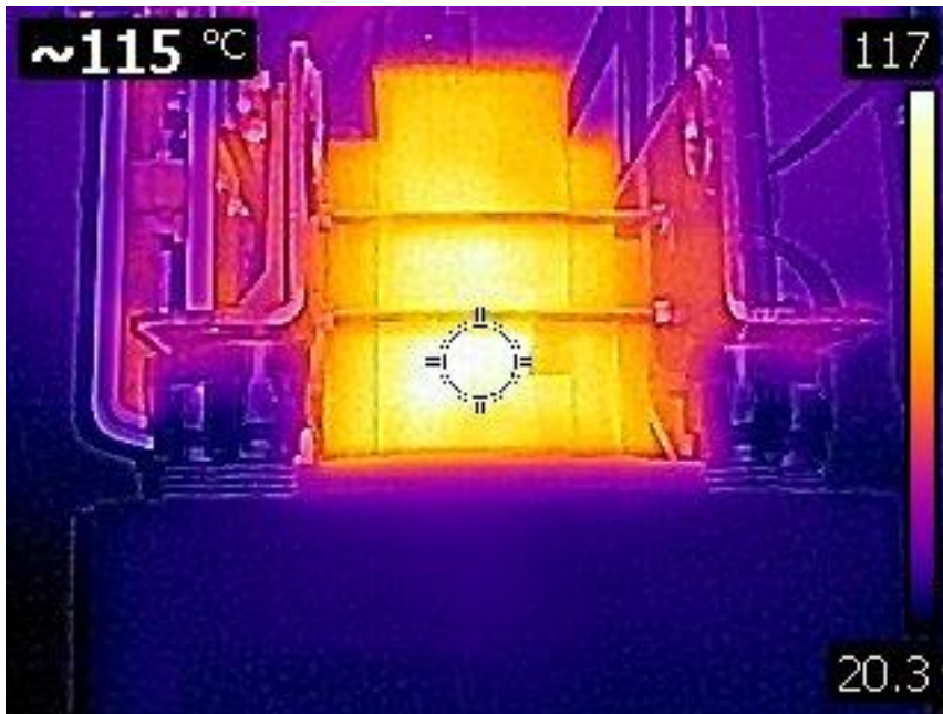
Fig. 15. Heating of the dry transformer magnetic circuit under the influence of harmonic distortion
